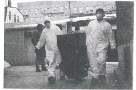
Members of the Youth Energy Corps carry a hopper for their blown-in insulation work.
